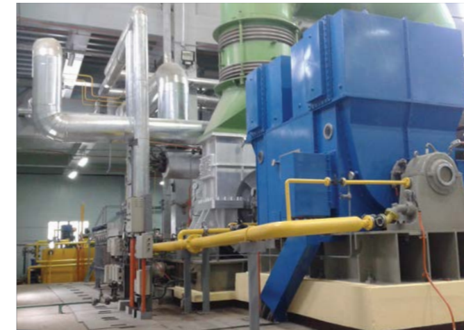
Waste Heat Recovery Facility
